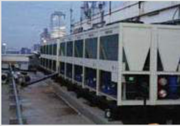
Instalasi AC Central
